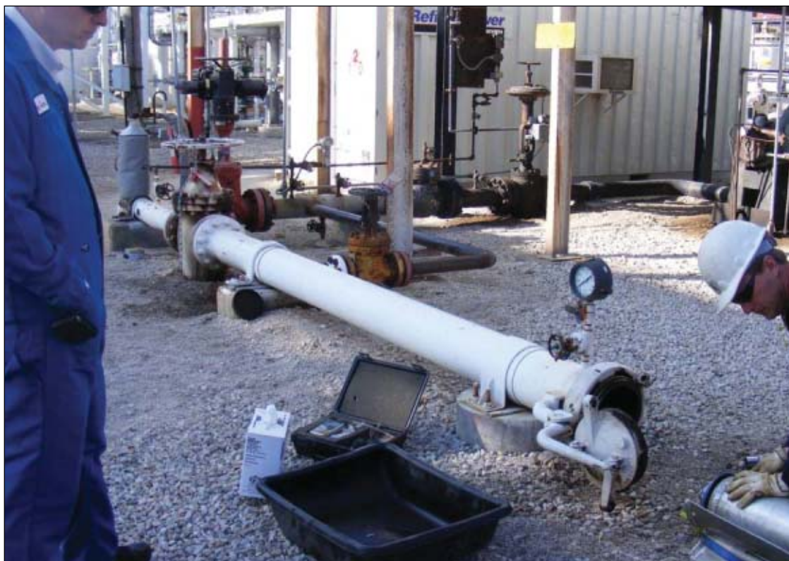
Technicians prepare to launch the tool into one of the Jayhawk products pipeline segments (Fig. 4).
